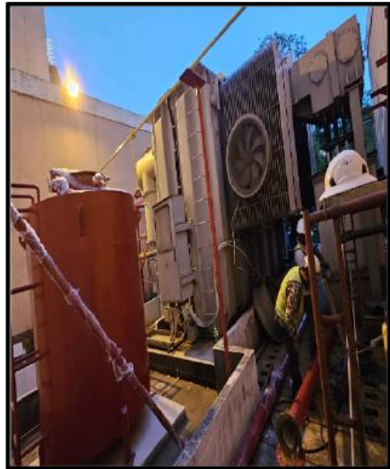
Location main tank
